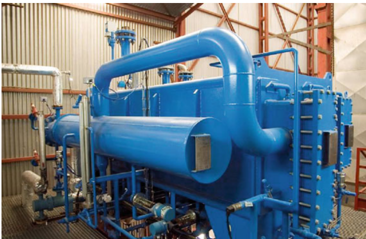
Fig. 1.10 Double-effect absorption heat pump located at the Plataforma Solar de Almería
