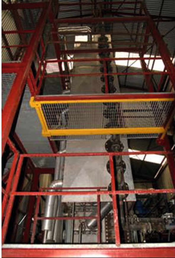
Fig. 3.1 Pilot MED plant located at the Plataforma Solar de Almería
