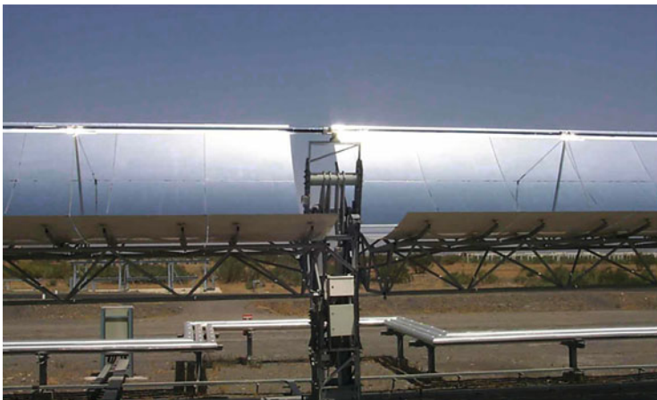
Fig. 4.3 Metallic structure onto which the parabolic-trough collector is mounted
