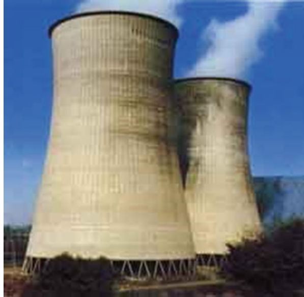
Fig. 2.17 Cooling towers in a CSP plant
