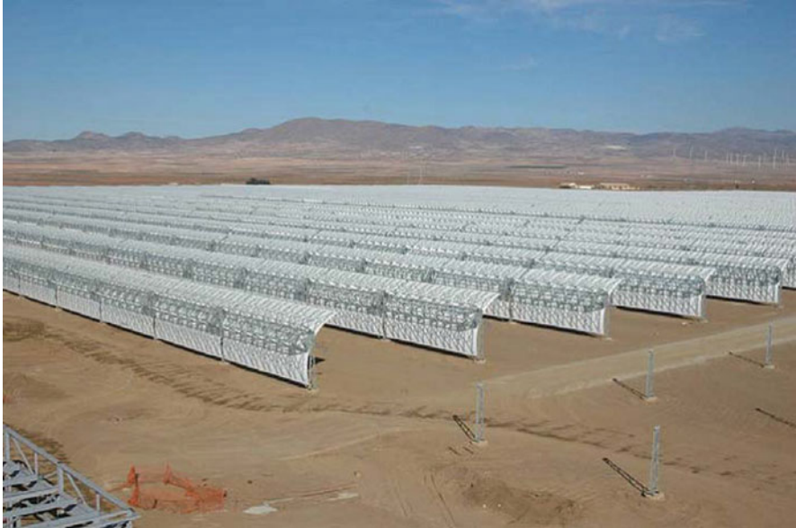
Fig. 2.15 Solar field of the Andasol-1 plant
