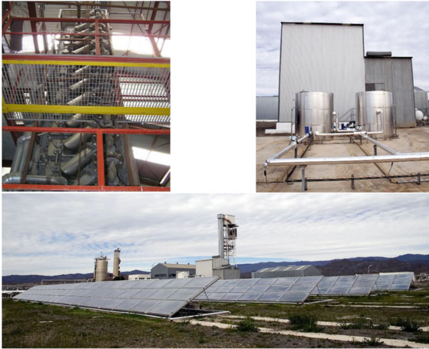
Fig. 1.8 Multi-effect distillation plant, storage system and compound parabolic collectors solar field at the Plataforma Solar de Almería
